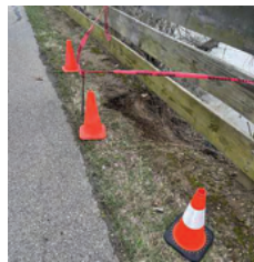
The Great Miami River Trail south of Crains Run Park is closed for several days while crews repair erosion. MIAMI CONSERVANCY DISTRICT / CONTRIBUTED
